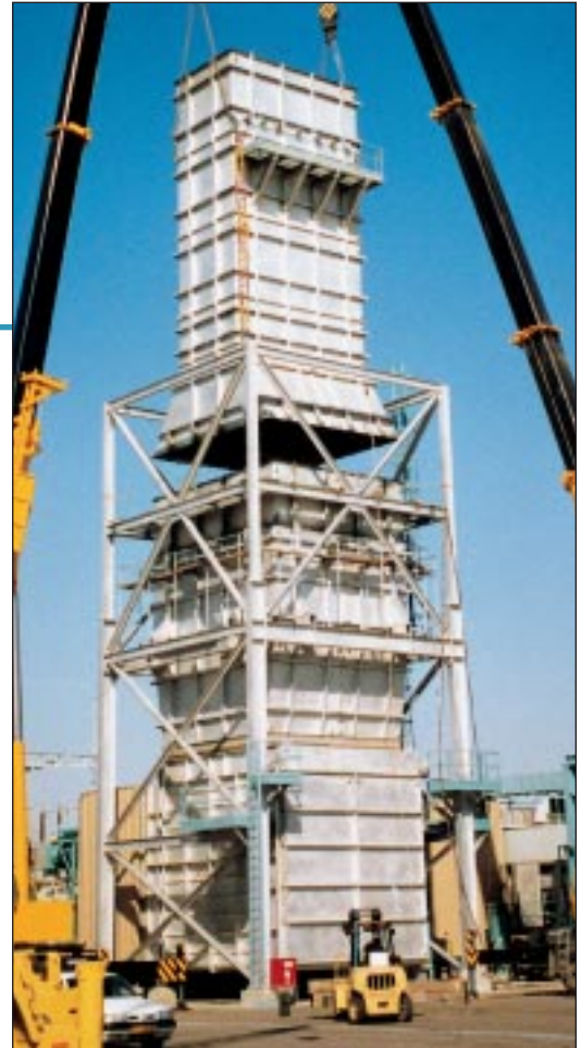
FS-9E inlet exhaust and silencing system.
