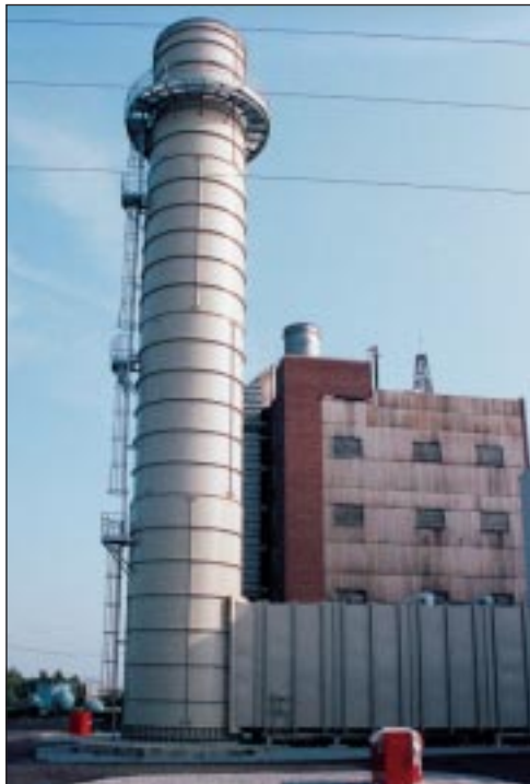
125' tall round stack for a W501-D5 turbine. Silencer panels are built into the horizontal ductwork leading into the stack.
